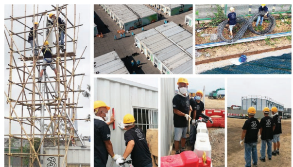
• The Group supports the construction of the shared network facilities at some community isolation and treatment establishments in Hong Kong.
