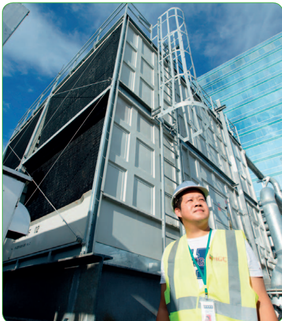
A dynamic cooling management system at an HGGC data centre reduces power consumed by air-conditioning.
