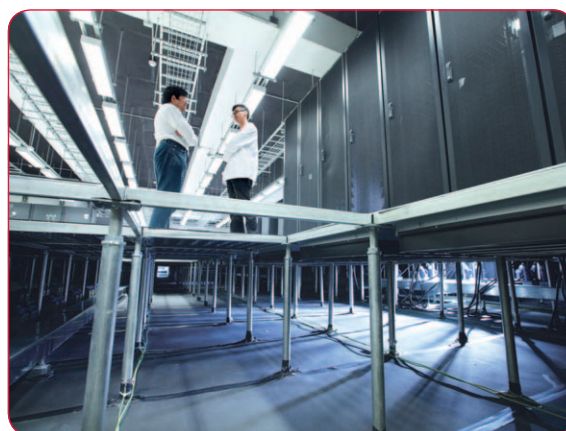
HGCGC provides enterprises with world-class server colocation, disaster recovery solutions and managed services.
